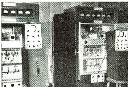
Dual transmitters installed at W2XVT for DuMont Labs., of Passaic, N. J.
